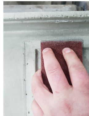
Ensure the flashing sits IN the recess of the tile over tray
